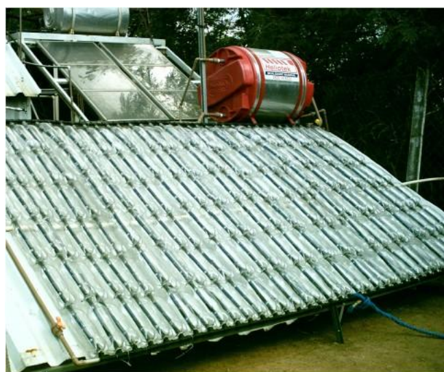
Figure 2. ASBC installed on Renewable Energy Center of UNESP, Guaratinguetá, SP. Font: (MORAES-SANTOS, 2015)
